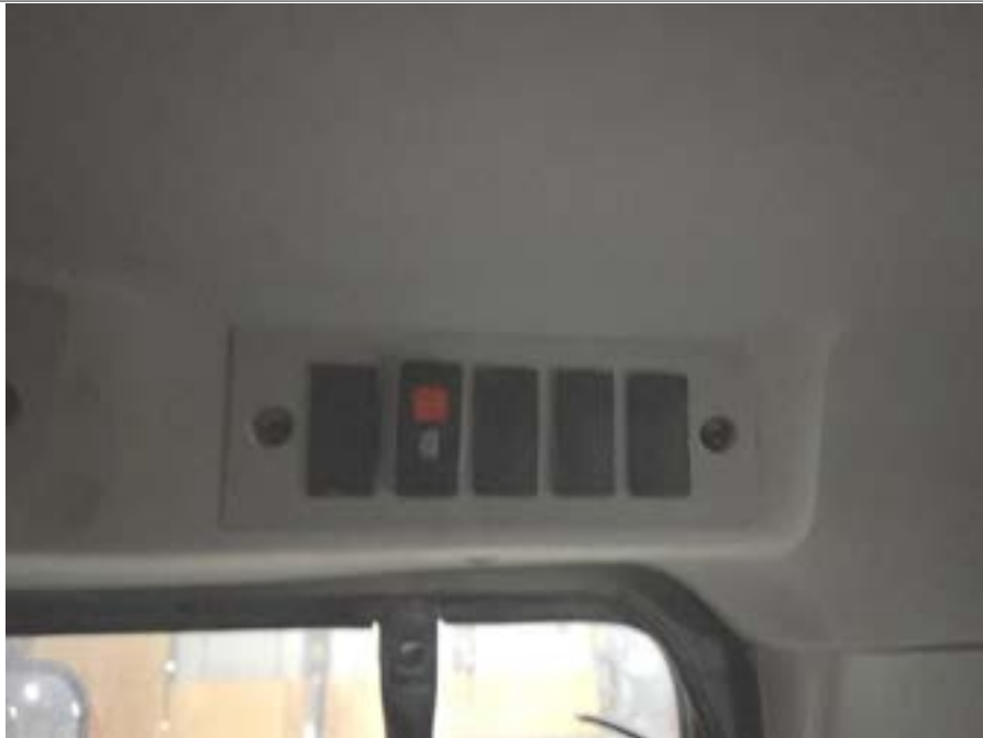
Switches and Controls
